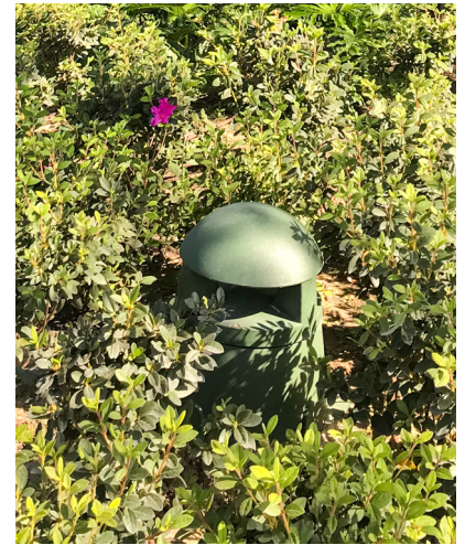
WEATHERPROOF GST-G SPEAKERS TUCKED WITHIN THE BEAUTIFULLY MANICURED LANDSCAPE ALONG WALKWAYS AND CONCOURSES
